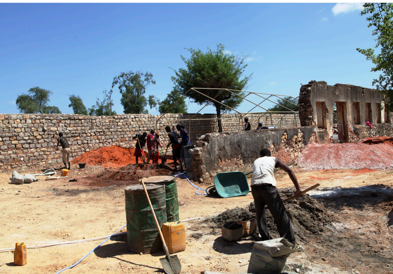
Baidoa's center of hope for misled youth under construction. UN Photo / Mahamud Hassan
