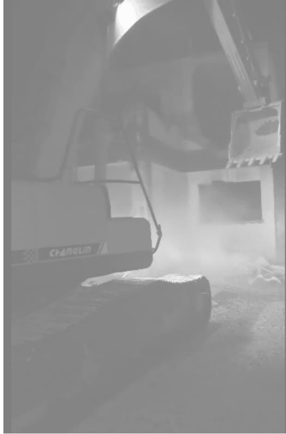
17 May 2024: Demolition of the Croix-des-Bouquets police station by 400 Mawozo Still from video shared with the Panel on 17 March
