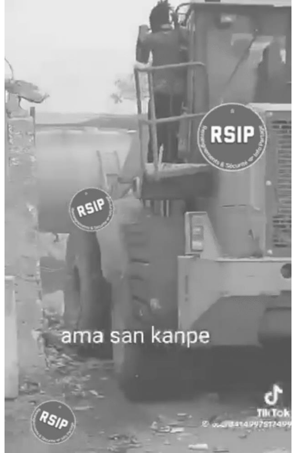
21 May 2024: 5 Segond demolishing the La Saline sub-station Still from video shared with the Panel on 22 March
